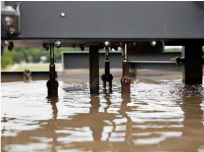
06/ FULL-LENGTH VALVE BRIDGE
